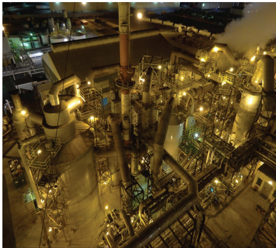
Ecoservices' Dominguez sulfuric acid plant recently replaced its converter's internal heat exchanger.
