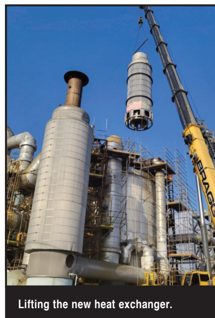
A new 55,000 lbs. heat exchanger made of 310SS is lowered into converter.
